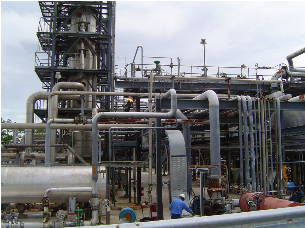
SE Gobe Production Facilities
