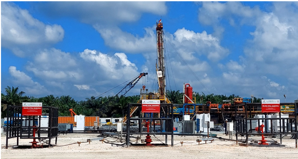
Wellheads and drilling rig at PB field, Mahato PSC
