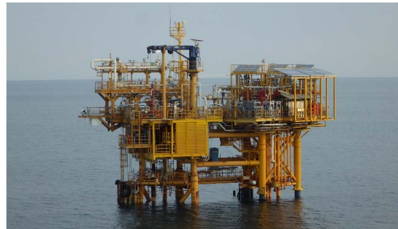
Oyong Well Head platform as a simplified gas production system.
